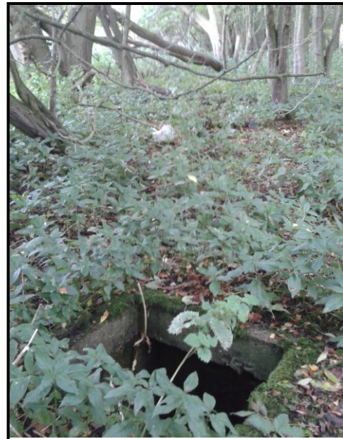
Figure 31: Man hole at site 4
